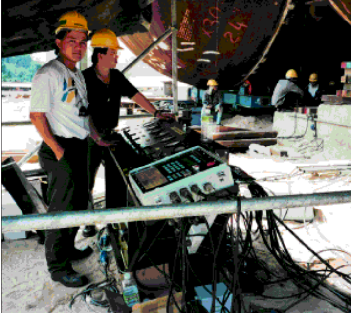
▼ Positioning of two enormous vessels, using a combination of stage and synchronized lifting in Malaysia.
